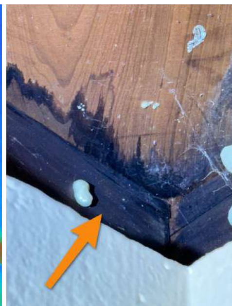
moisture intrusion stains
