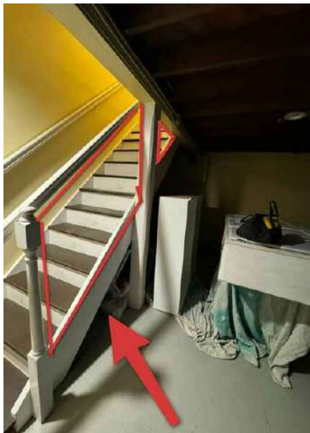
Large gaps not safe for small children
